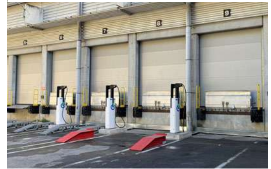
Figure 7: Depot charging (Kirkland, WA) (Source: Chargepolly)
