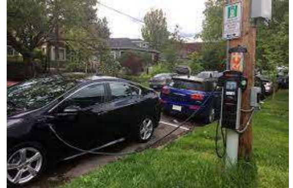
Figure 12: Metered curbside charging (New York City)
