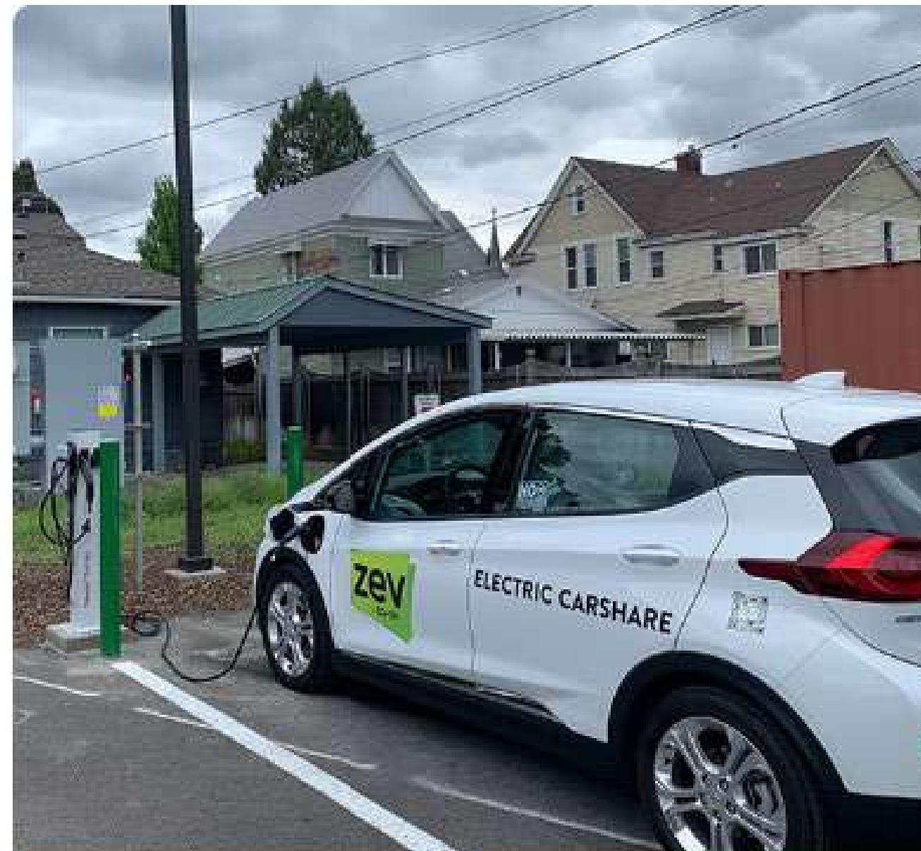
A new charging station at the GU Office of Sustainability
