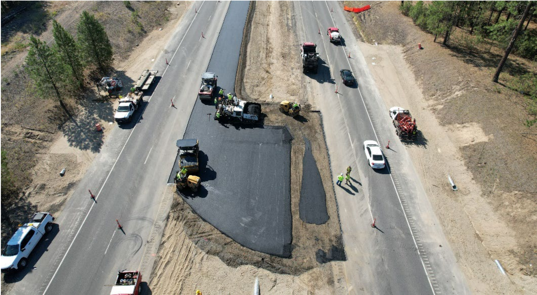
J-Turns added at US 2 & Colbert Road in north Spokane after several serious and fatal collisions.
