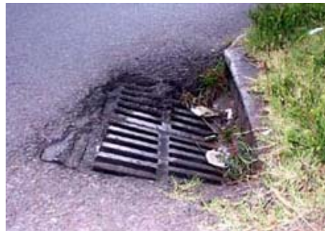
Poorly maintained drainage grate
